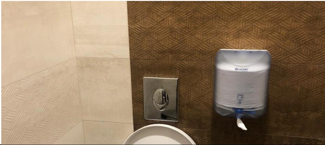
Dual toilet flush
